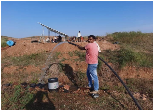
Working Solar pump
